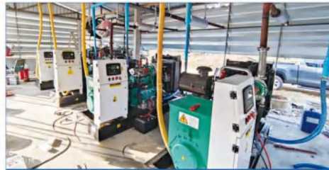
Thailand 7 Units Biogas Generator Set
