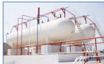
Gas Centralized Supply
