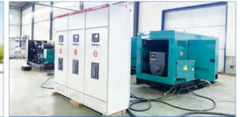
Mexico Paralleling 200kWx2 Natural Gas Generator Set
