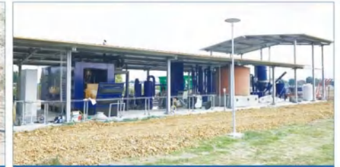
Italy 200kW Biomass Gasifier System
