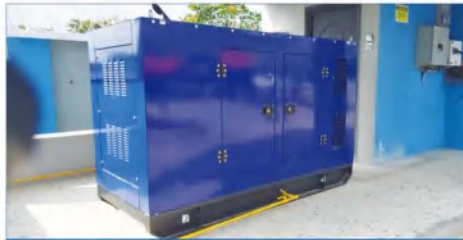
Nigeria 13 Units LPG Generator Set
