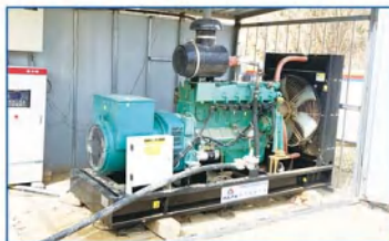
Power Generator for self use or to the grid
