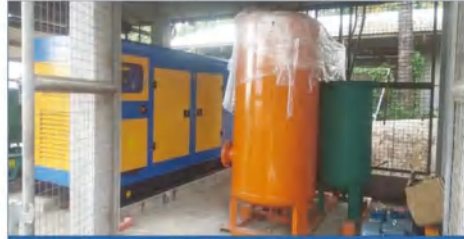
Philippines 150kVA Biogas Generator Set
