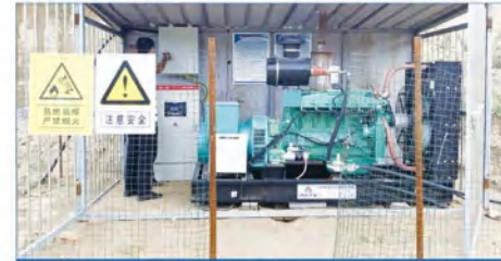
China Oil Associated Gas Generator Set
