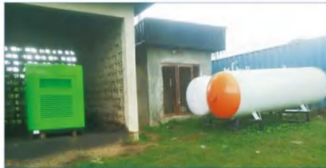
Nigeria 5 Units LPG Generator Set
